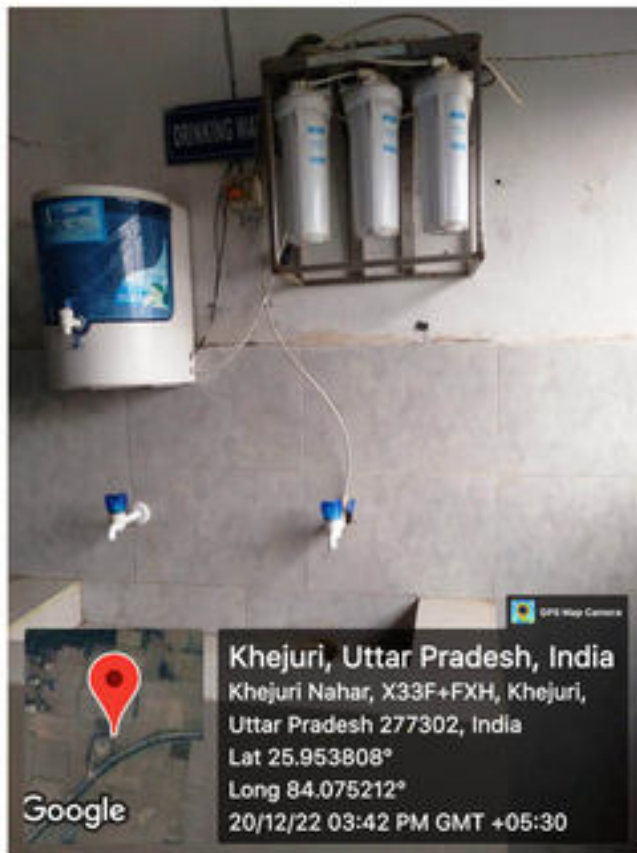
Drinking Water Facility
