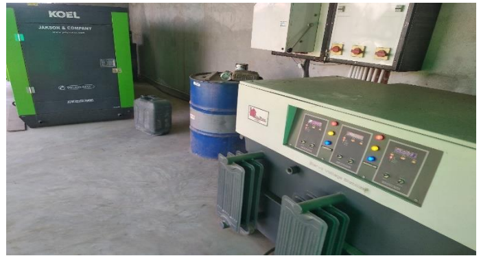
Power Backup System
