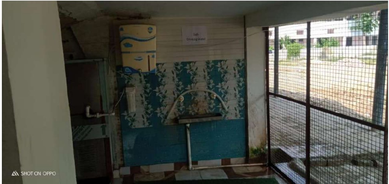
Fresh Drinking Water
